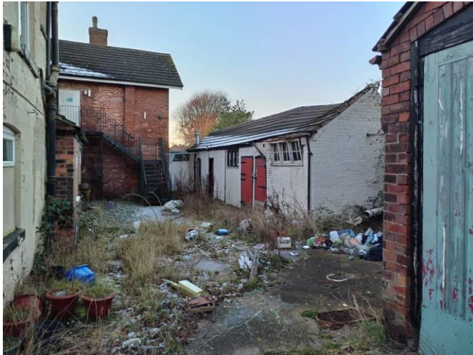
The rear of the dilapidated building boarded up in part, with dispersed litter and fly tipping.
